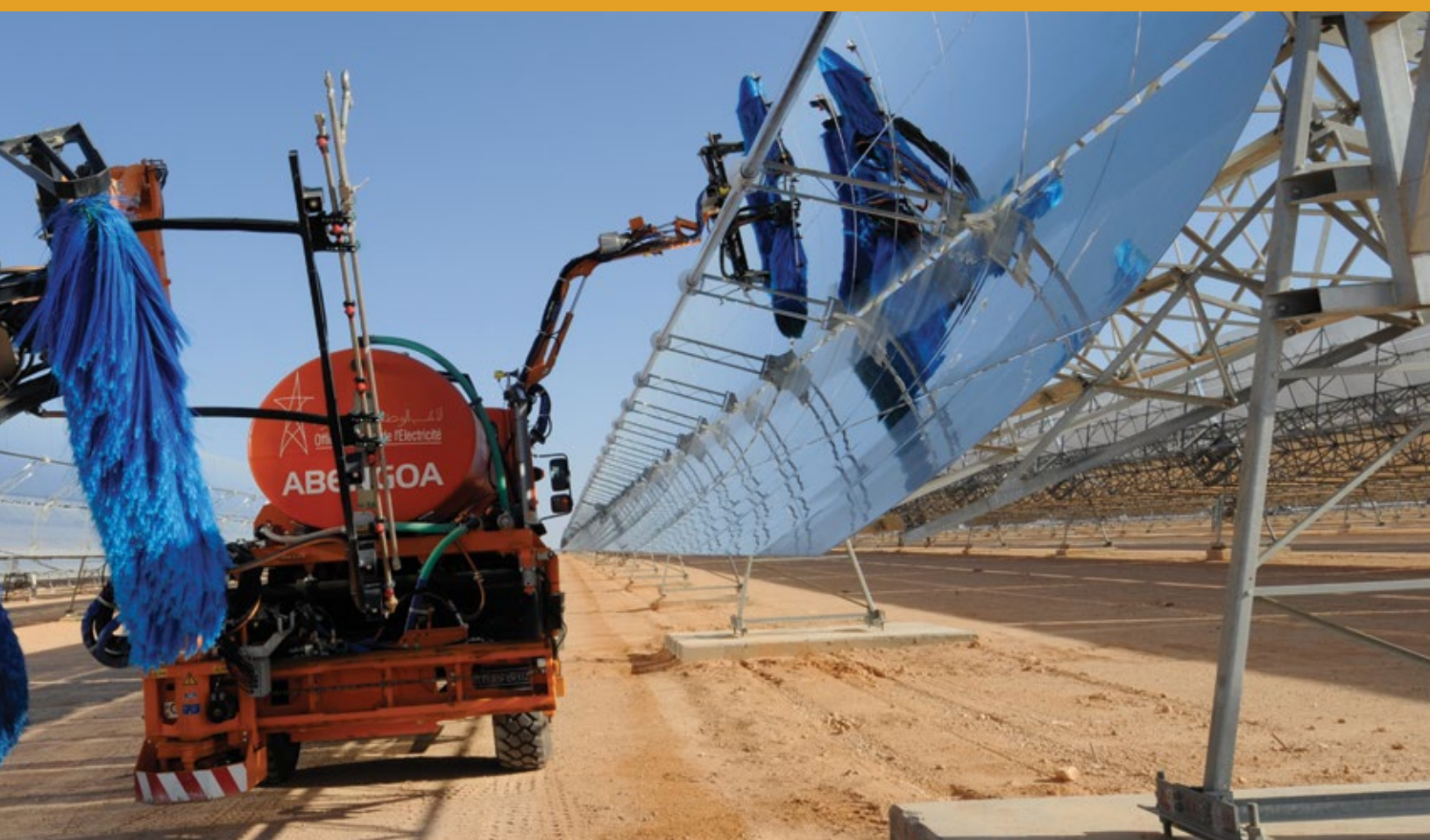
Combined Cycle Thermo-Solar Power Plant in Morocco. © World Bank/Dana Smillie
