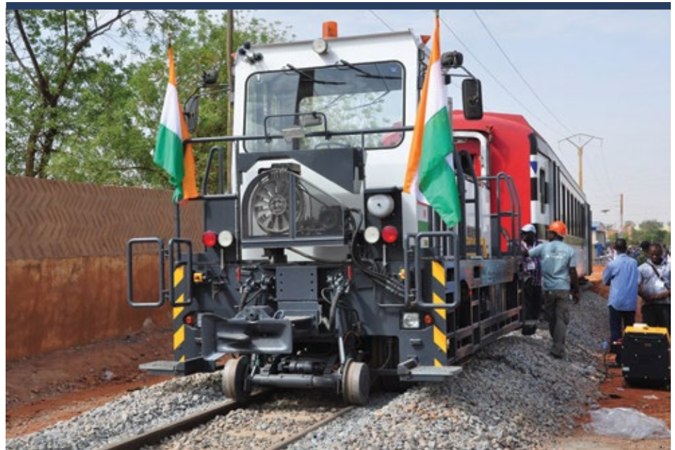
Workers lay rails at a train station outside Niamey, Niger. © Ado Youssouf
