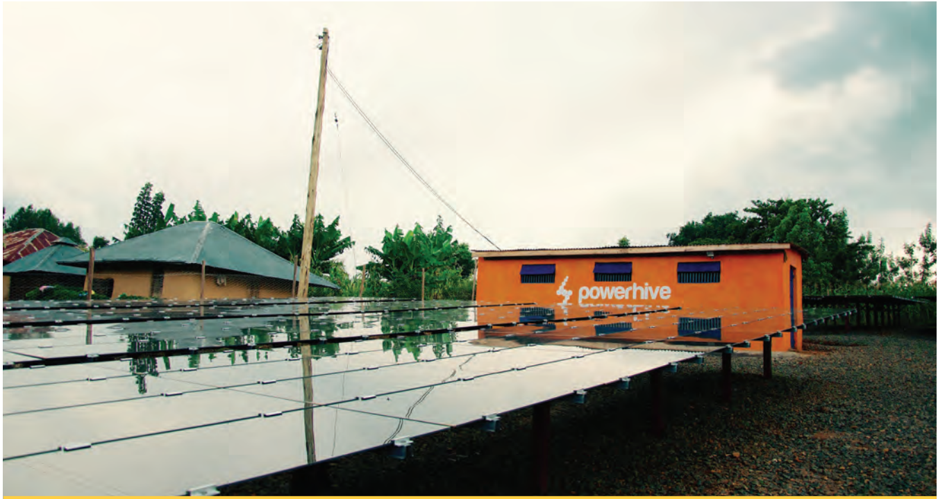
Powerhive – 100% solar off-grid microgrid in Western Kenya.
