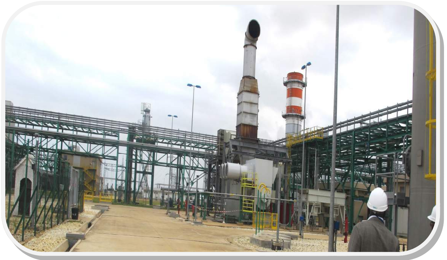
Congo Power Plant - Pointe-Noire
